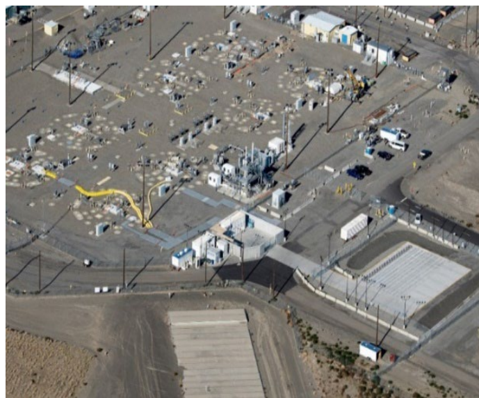
AP Tank Farm and Tank-Side Cesium Removal System
