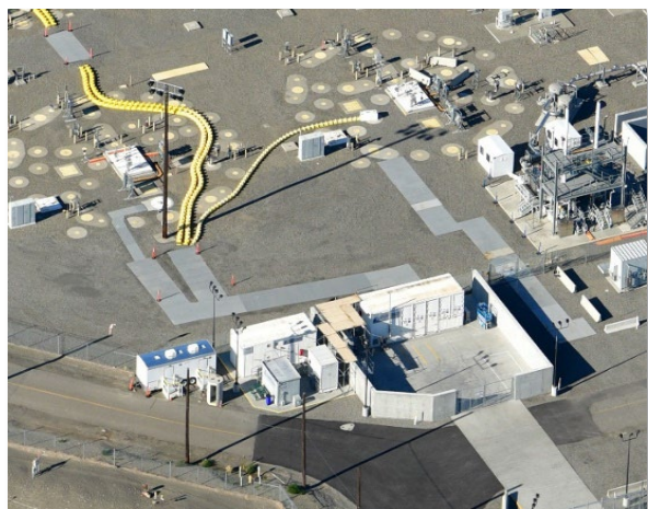
Tank-Side Cesium Removal and AP Tank Farm
